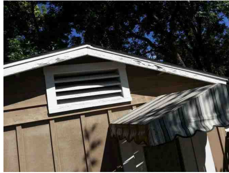
Exterior Trim Peeling Paint
